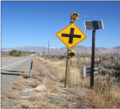
Figure 2. Solar power advanced warning flasher installed NB and SB on SH-75.
