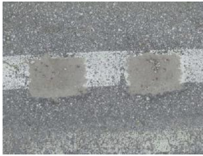
Rumble stripe with caked material and debris in the bottom
