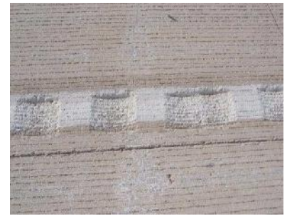
Similar wear for edge line in rumble stripe and flat section
