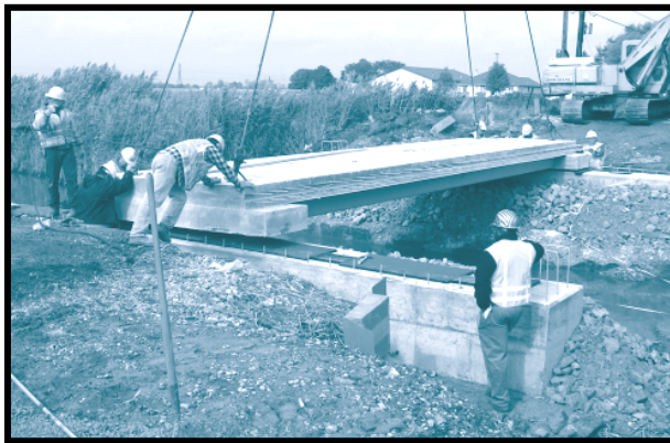
Monroe County Road Commission maintenance workers place a precast deck slab for the new Suder Ave. Bridge.
