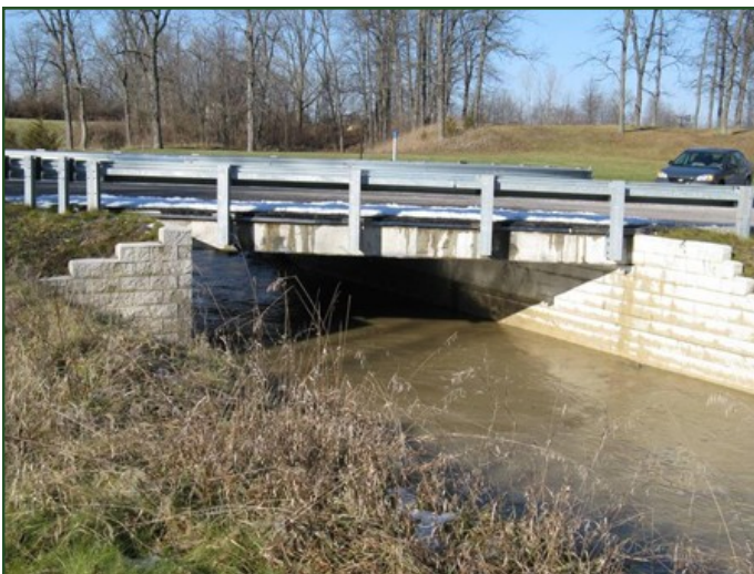
Bridges built using the Geosynthetic Reinforced Soil Integrated Bridge System (GRS-IBS) include the Vine Street bridge in Defiance County, OH.
