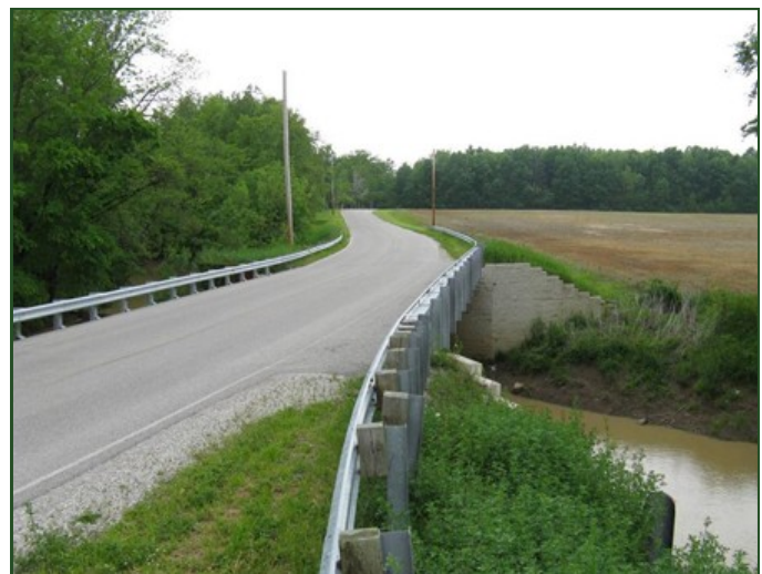
The Bowman Road bridge in Defiance County was the first bridge in the world to use GRS-IBS.
