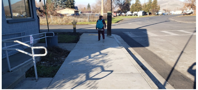
City of Lapwai: Main Street Sidewalk & ADA Ramp Phase II—Before, During, and After
