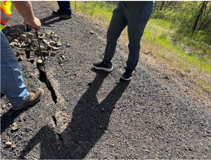
Measuring one of the voids under the road surface.
